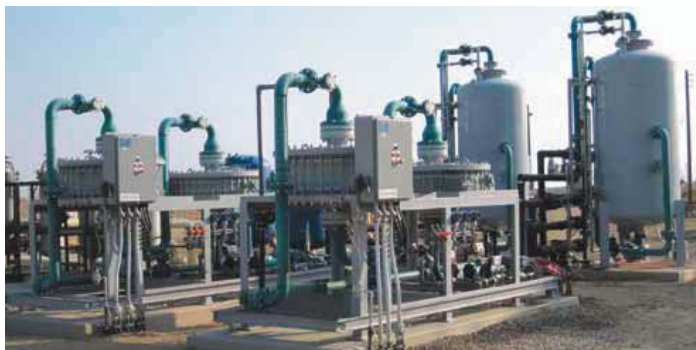
Produced water treatment system in Maricopa, California, with Spectrum Plus Micro-Media Filters and RecoPur SAC/WAC Ion Exchange Softeners.
